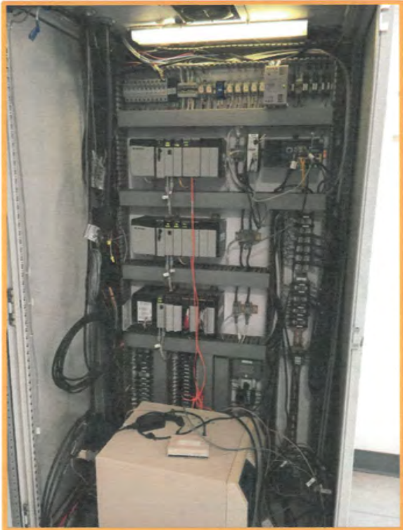
Rockwell Motor Control Center
