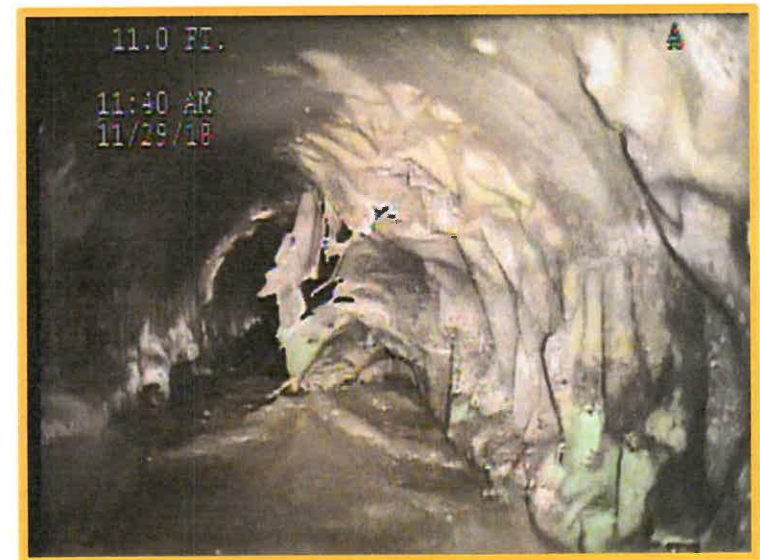
Cucamonga Trunk Sewer Coating Failure
