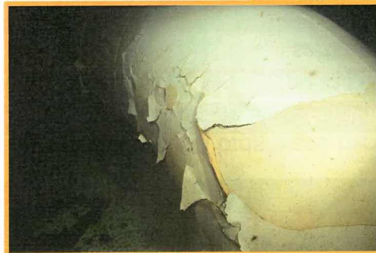
Coating Delamination on Piping
