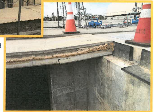
Concrete Cover Failure
