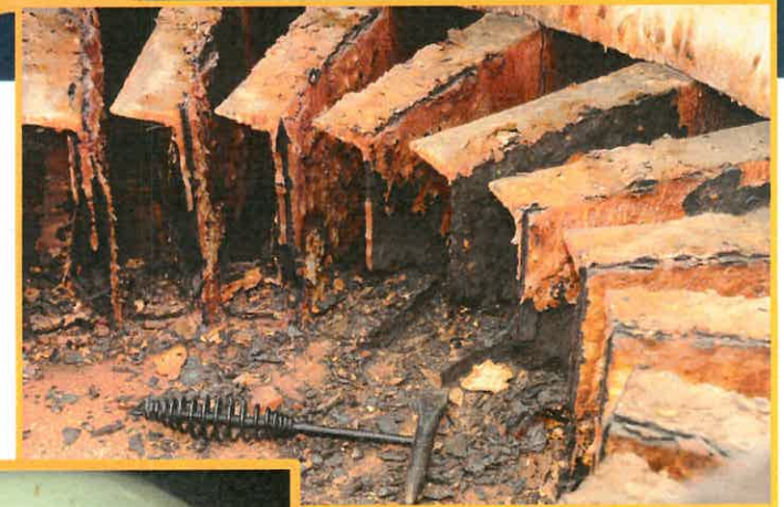
Corrosion Damage on Rafters
