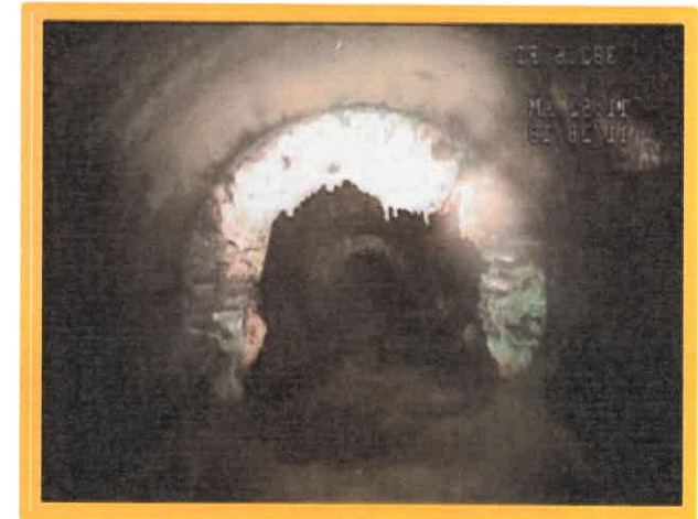
Cucamonga Trunk Sewer Coating Failure
