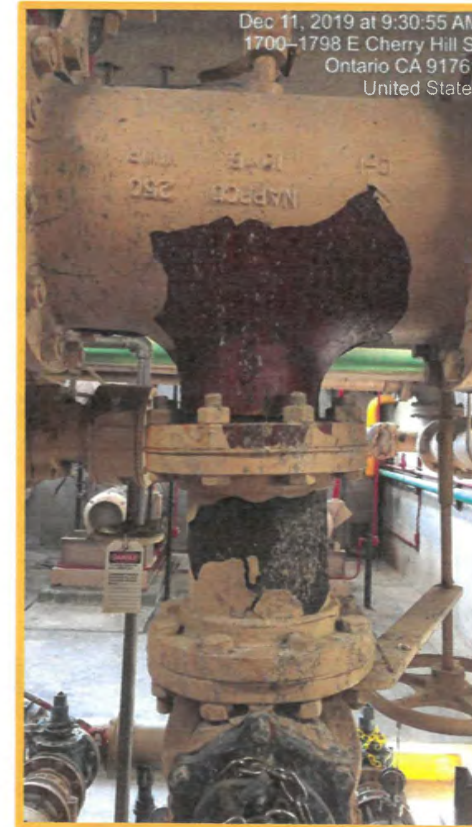
Failed Sludge Pipe 2
