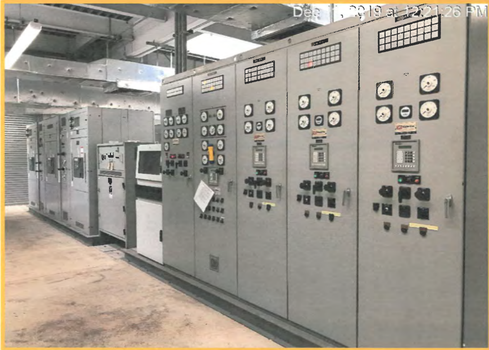
RP-1 Emergency Generator Control Panels
