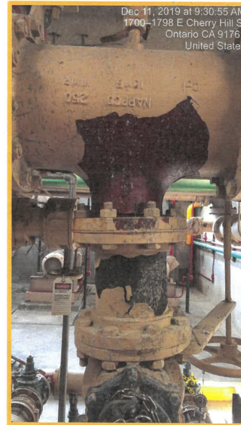
Failed Sludge Pipe 2
