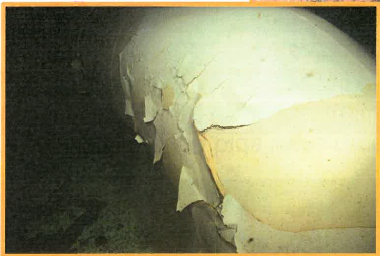
Coating Delamination on Piping
