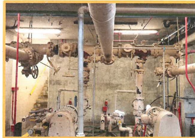
Ruptured Primary Sludge Piping
