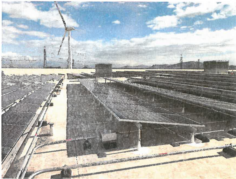
The new 1.5 MW solar panels at IERCF installed by AMS.
