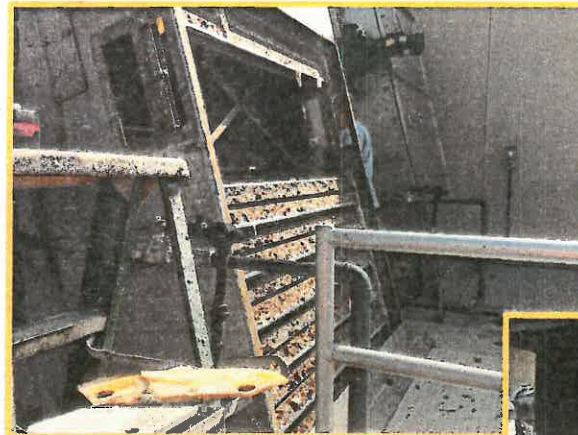
Exposed Fine Screens
