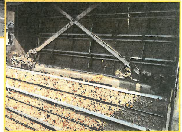
Rag Accumulation Inside Fine Screens
