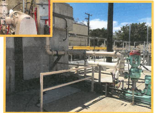
Grit Pump Discharge Pipeline
