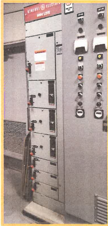
RP-1 SCADA MCC
