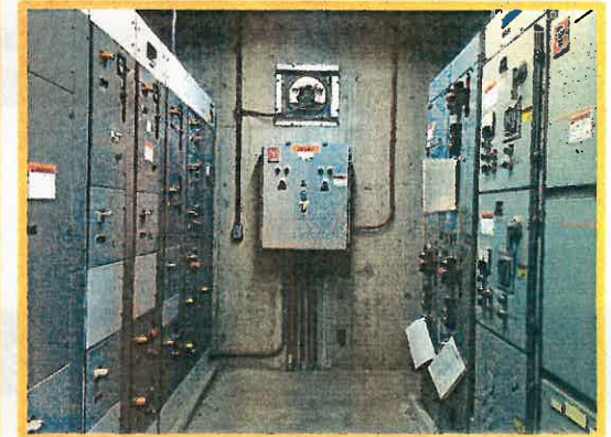
Existing Motor Control Center
