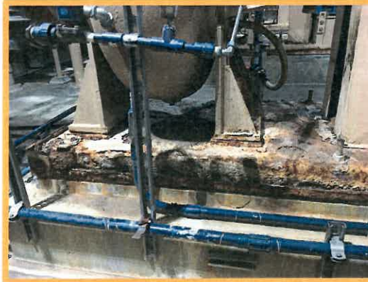
Corroded Sludge Pump Base
