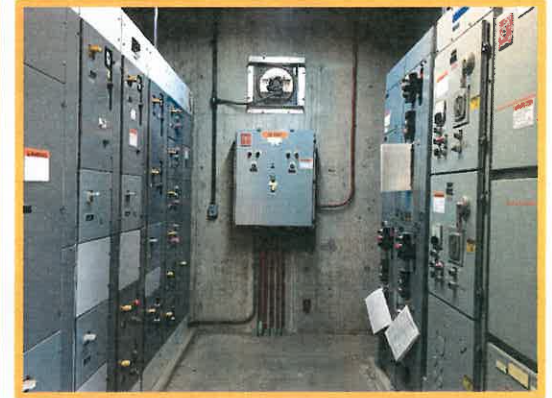
Existing Motor Control Center
