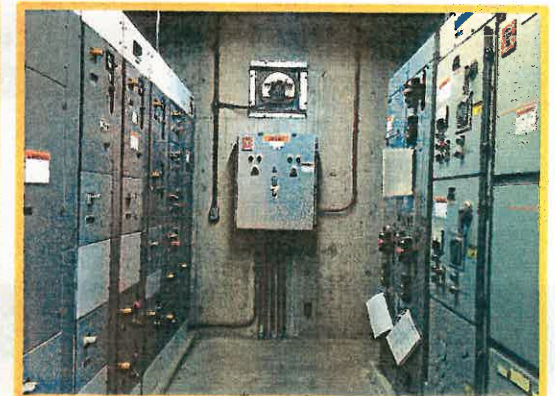
Existing Motor Control Center
