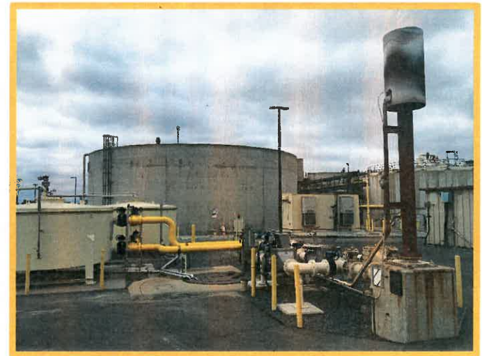
RP-1 Existing Flare System
