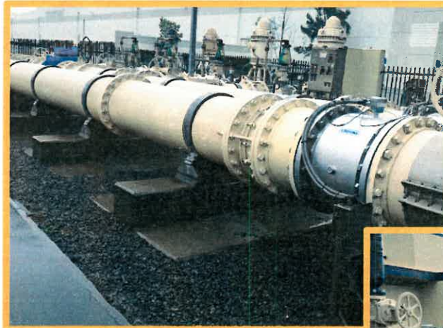
San Bernardino Lift Station Force Mains
