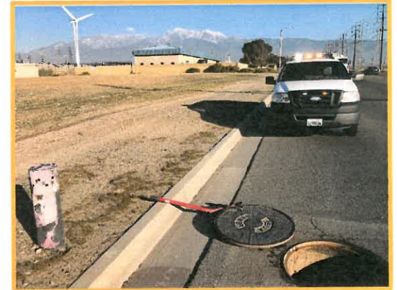
Air Relief Valve in Etiwanda Ave.
