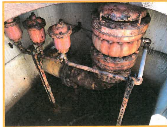
Air Relief Valves to be Replaced
