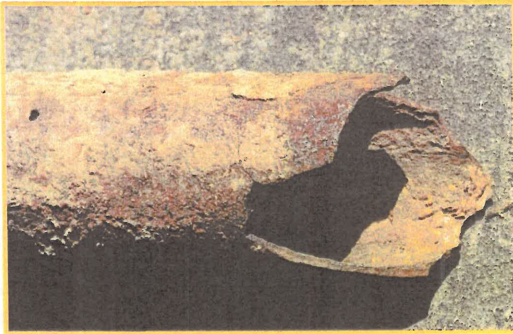
Example of Extremely Corroded Pipe
