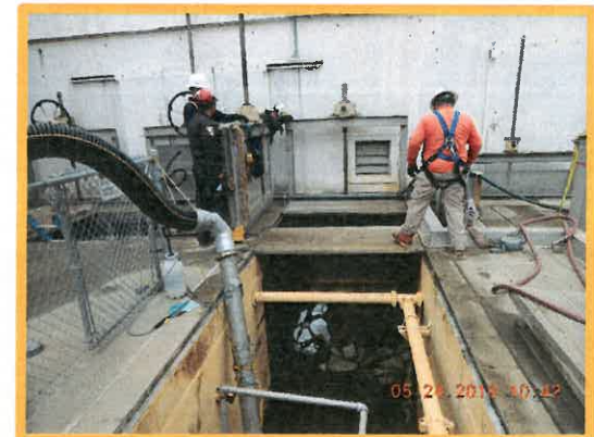
Contractor attempting to manage Leakage
