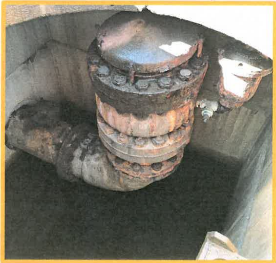
Existing Combination Air Relief Valve
