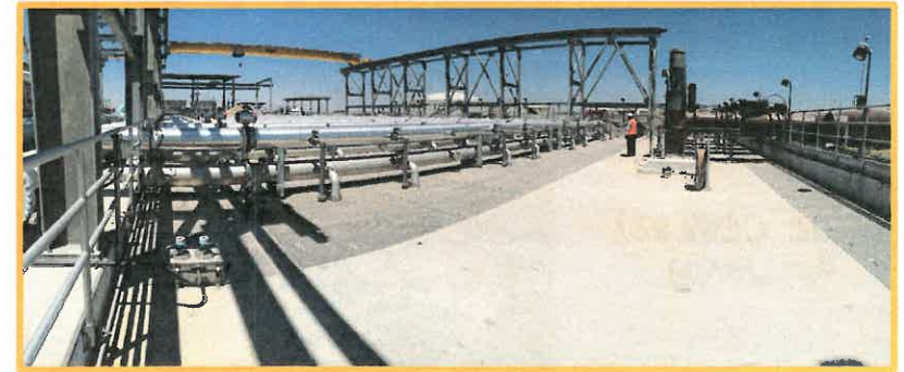
Visalia Water Recycling Facility Suez Membrane Bio-Reactor System
