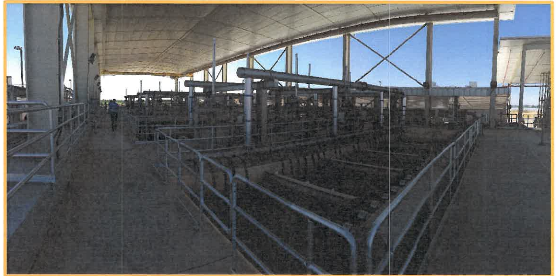
City of Modesto MBR System
