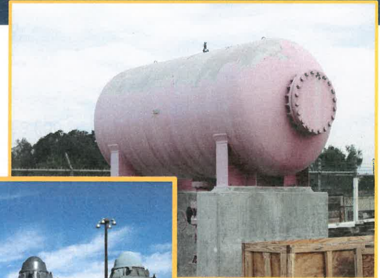
Existing 2,500 Gallon Surge Tank
