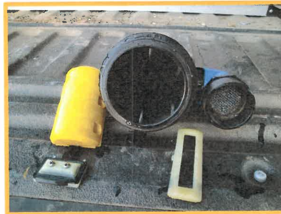
Inside existing A.R.I. Valve
