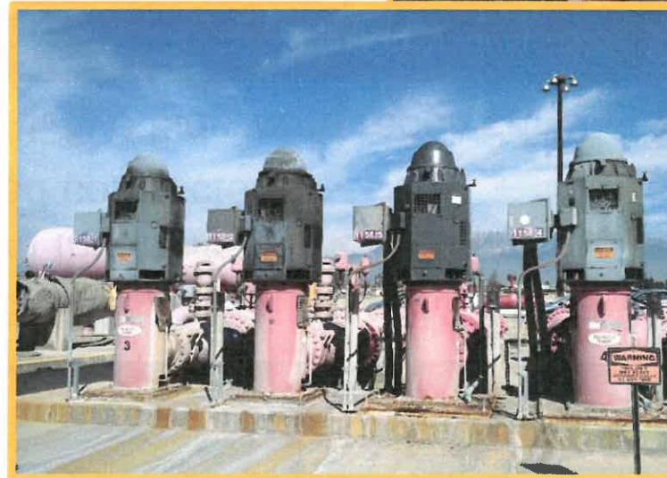
RP-1 Recycled Water Pump Station
