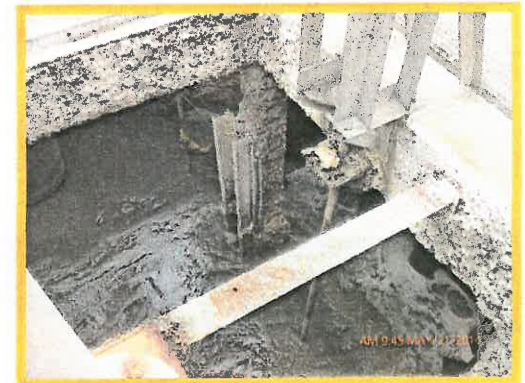
Distressed Diversion Structure
