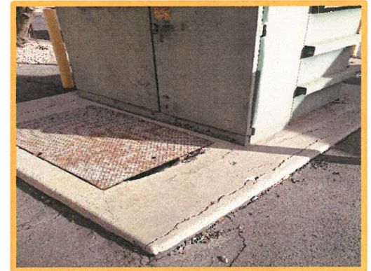
Spalled Concrete Transformer Pad
