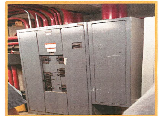
Distribution Panel at T-Plant Basement
