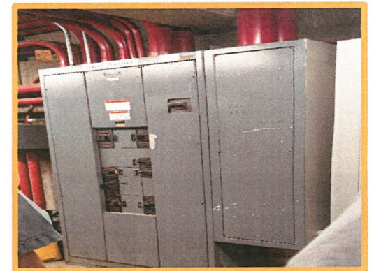
Distribution Panel at T-Plant Basement
