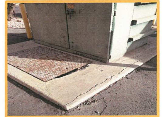
Spalled Concrete Transformer Pad
