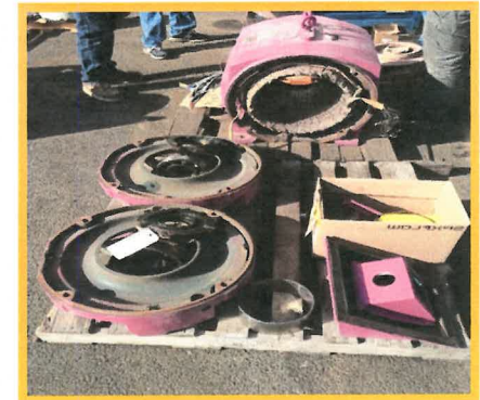
1050 RW Pump No. 2 Disassembled at the Contractor Shop
