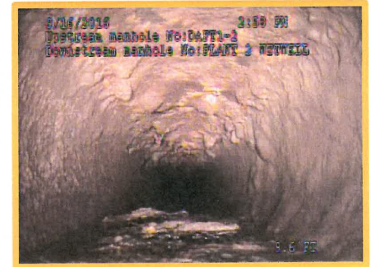
Buildup in 18" Subnatant Pipeline
