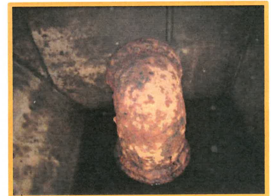
Corroded Pipe in Pump Station Wet Well
