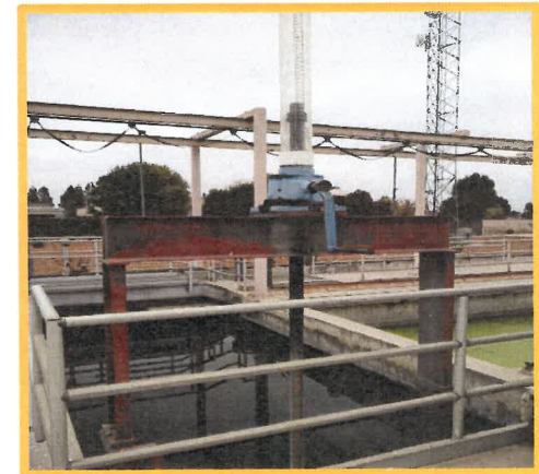
Corroded Isolation Gates at the Filters
