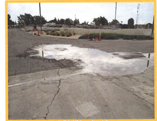
Surface Cracks and Drainage Issues
