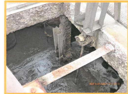
Exposed Rebar in Grating at Support Beam
