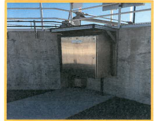
New Control Panel
