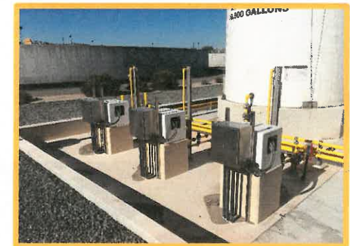
New Chemical Pumps
