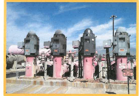
RP-1 1158 RWPS 400 HP Pumps
