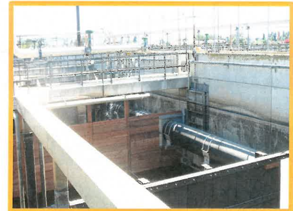
Baffle Walls and Mixed Liquor Return Pumps Pipe
