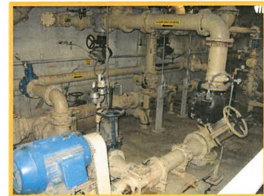
Existing Scum System
