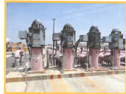
Recycled Water Pump Station Motors
