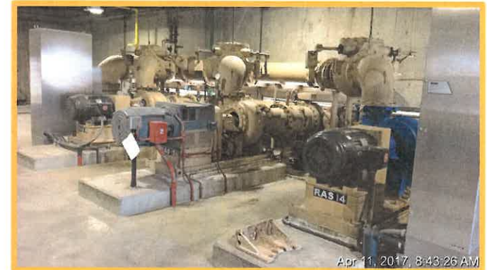
RAS Pump Equipment and Appurtenances
