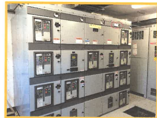
Front of Switchgear
