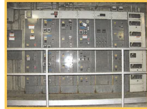
Obsolete Electrical Components
