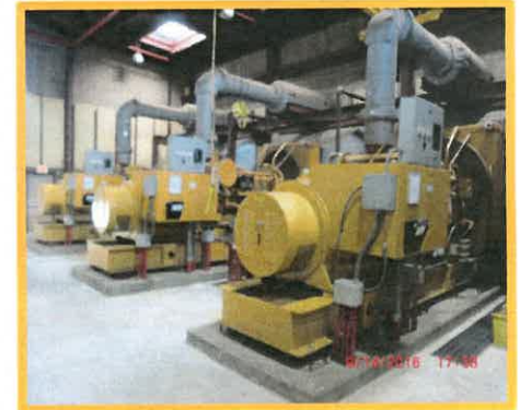
Back up Generators at RP-1
