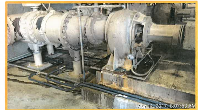
RAS Pump at End of Useful Life
