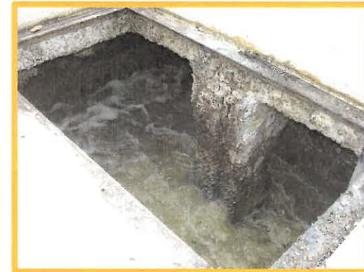
Corroded Concrete Deck
