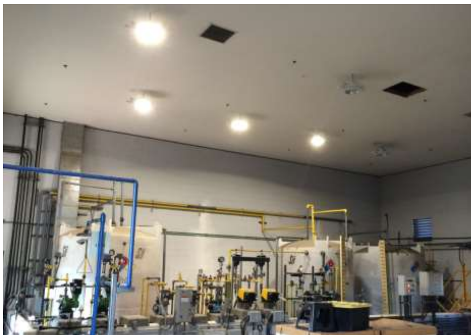
LEDs installed at RP4's chemical storage room
