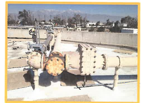
Digester No. 6 Flame Arrestor
