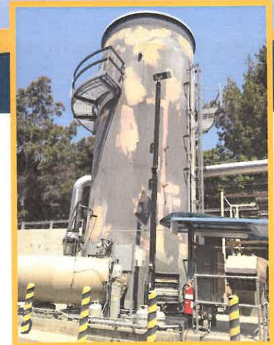
LACSD Flare (Site Visit)
