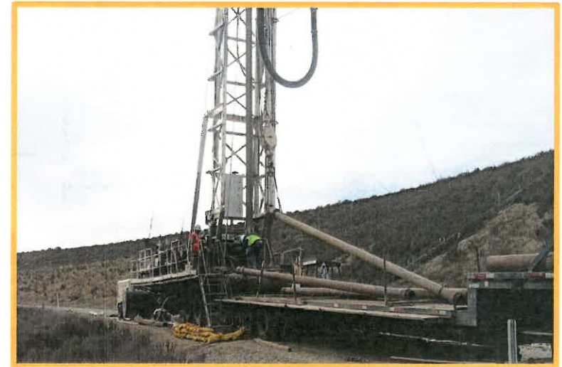
Past Construction of a Monitoring Well for San Sevaine Basin South End of Basin 5
