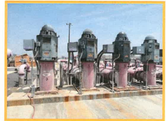
Recycled Water Pump Station Motors
