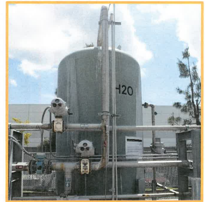
Deterioration of Surface Coating on Process Vessel
