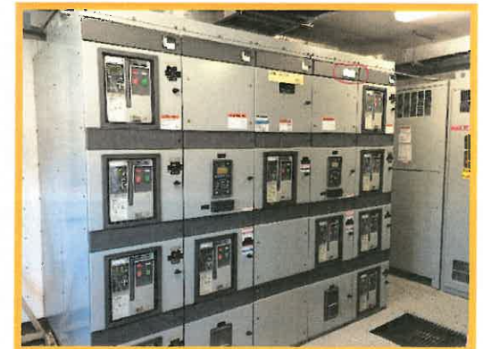
Front of Switchgear
