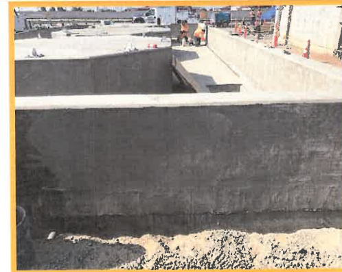
New Chemical Area with Tank Pad
