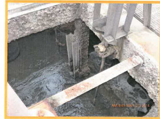
Exposed Rebar In Grating at Support Beam
