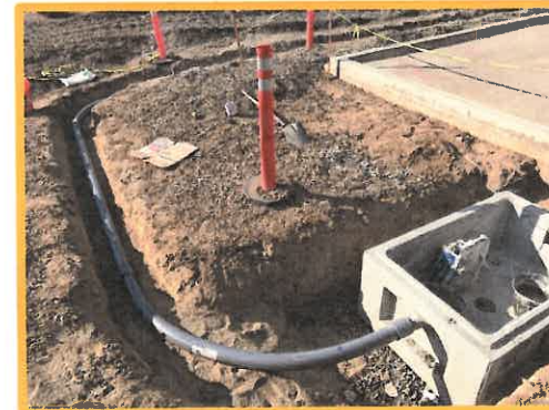
New Chemical Piping and Pull Box
