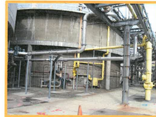
Above-Ground Connection at Digester 1
