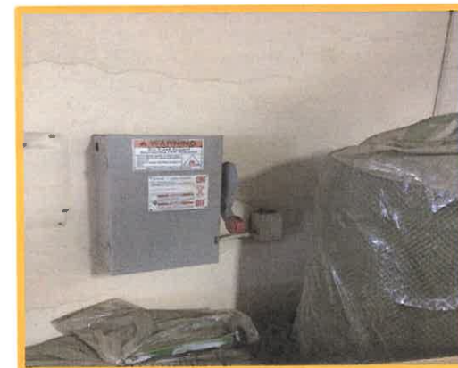
Disconnect to be Removed
