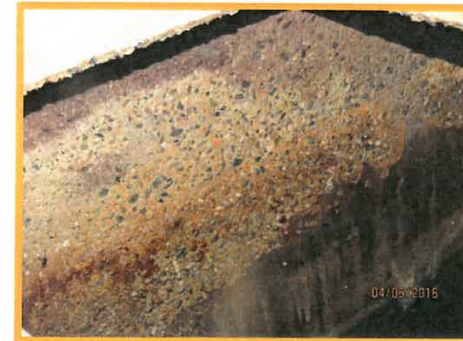
IPS Wet Well Concrete Corrosion
