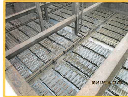
Drained Aeration Train No. 2
