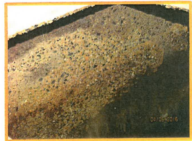
IPS Wet Well Concrete Corrosion
