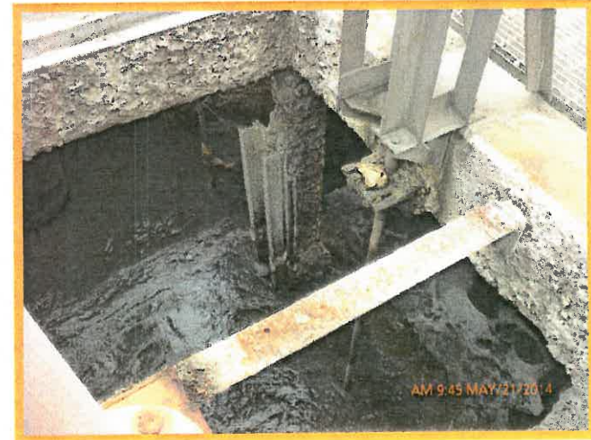
Exposed Rebar In Grating At Support Beam
