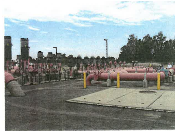
RP-1 Recycled Water Pump Station
