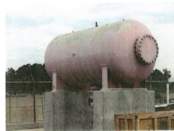
Non-operational surge tank
