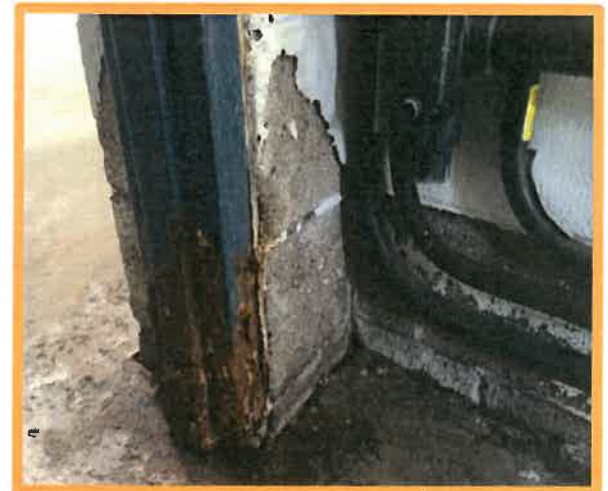
Corrosion from Bleach Leakage
