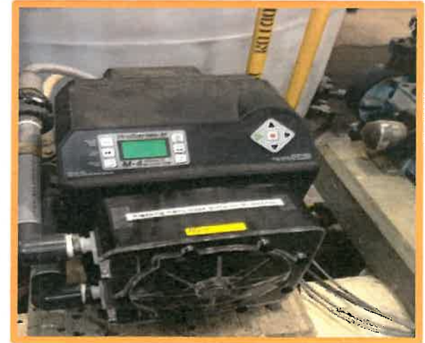
Existing and Old Diaphragm Pump
