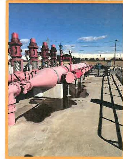
Pump Station Header
