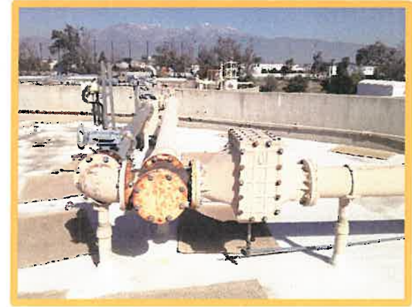
Digester No. 6 Flame Arrestor
