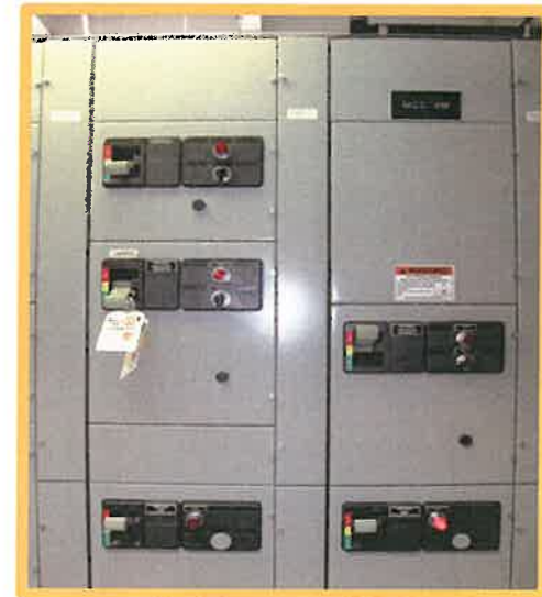
Switchgear at RP-1
