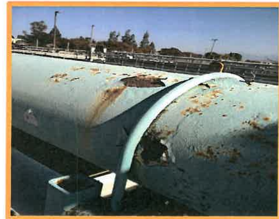
Rusted Pipe Surfaces
