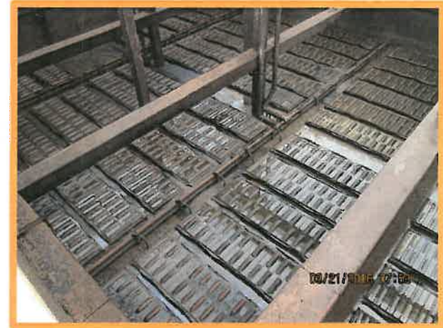
Drained Aeration Train No. 2
