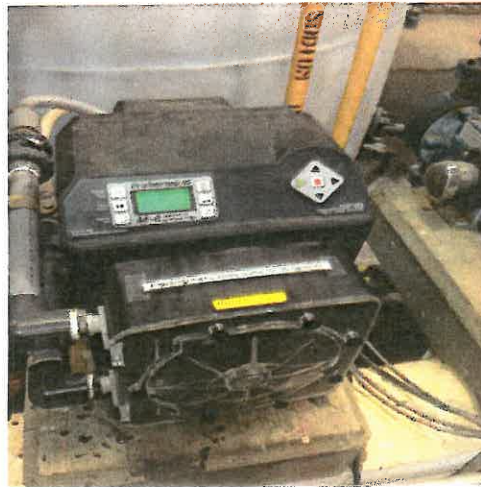
Existing Diaphragm Pump
