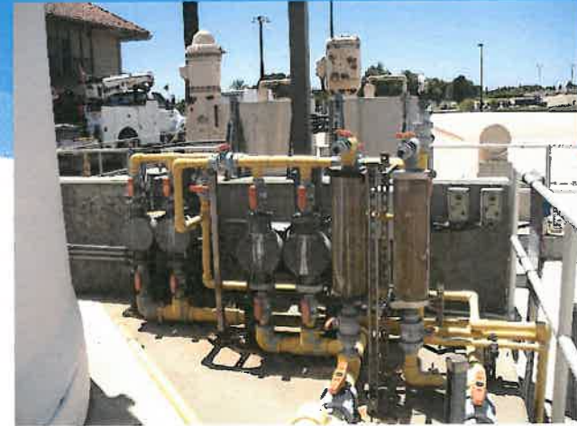
Existing TP-1 FM-1 Bleach Pumps
