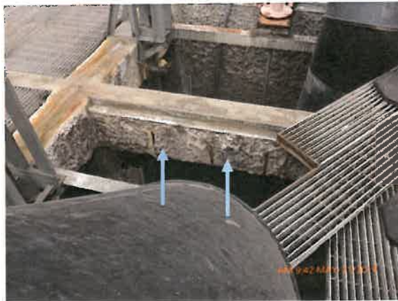
Exposed Rebar in Grating in Support Beam
