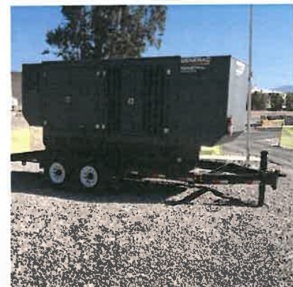
Existing Portable Generator
