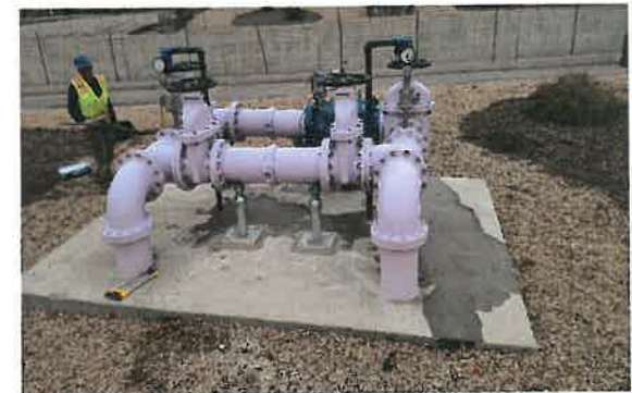
Completed RP-1 Utility Water Flow Meter
