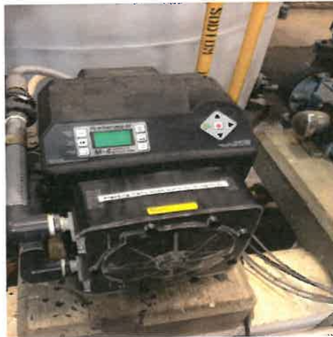
Existing Diaphragm Pump
