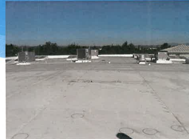
Existing Deteriorated TPO Roof Membrane
