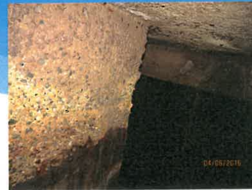
Intermediate PS No. 2 Concrete Degradation & Exposed Aggregate in the Vapor Space
