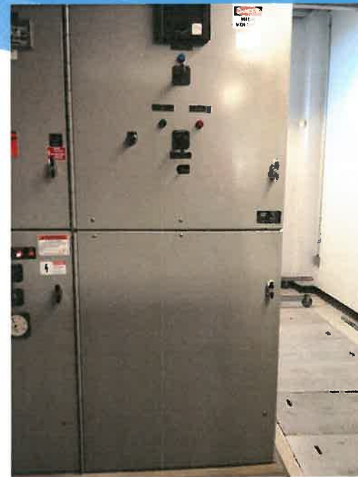
Vertical Switchgear Inside the Power Reliability Building
