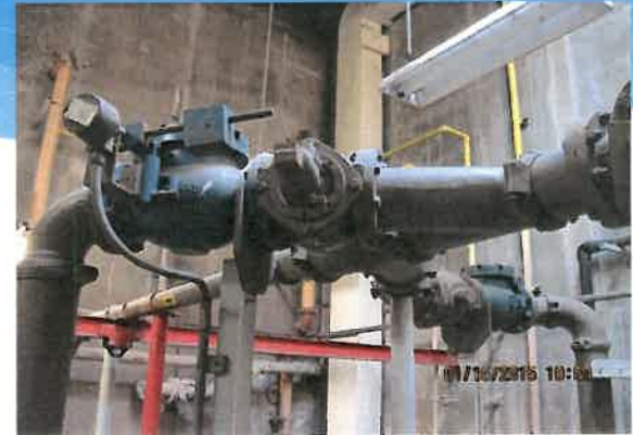
Existing Plug Valves
