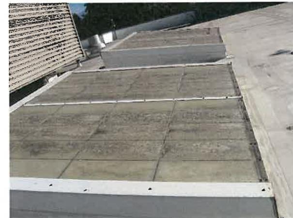
Discolored and Delaminating Skylight
