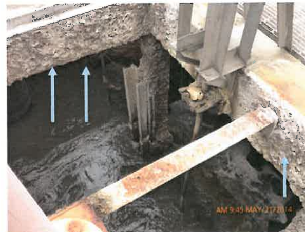
Primary Effluent Splitter Box Weakened Concrete and Section Loss
