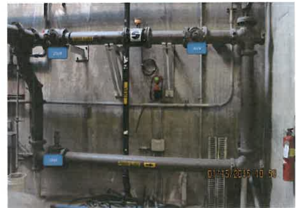
Primary Sludge Pipes
