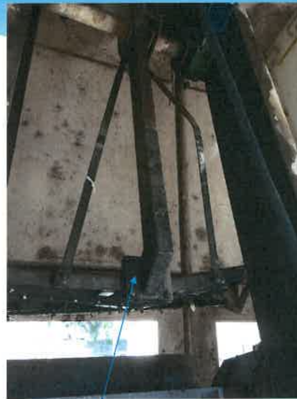
Bar Rake Frame Assembly Damaged and Refurbished
