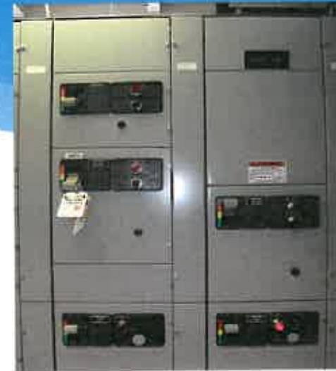
Switchgear at RP-1
