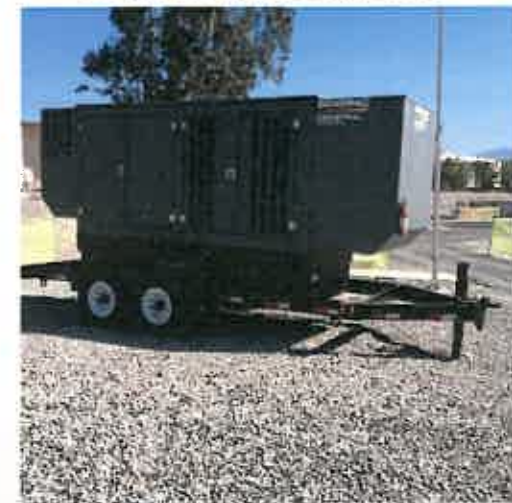
Existing Portable Generator
