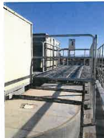
HVAC Unit Platform
