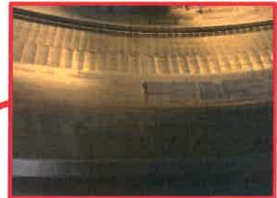
Close up of bearing housing surface damage
