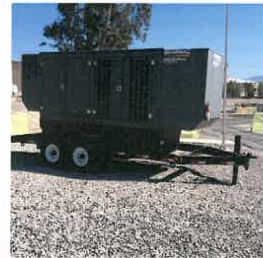
Existing Portable Generator
