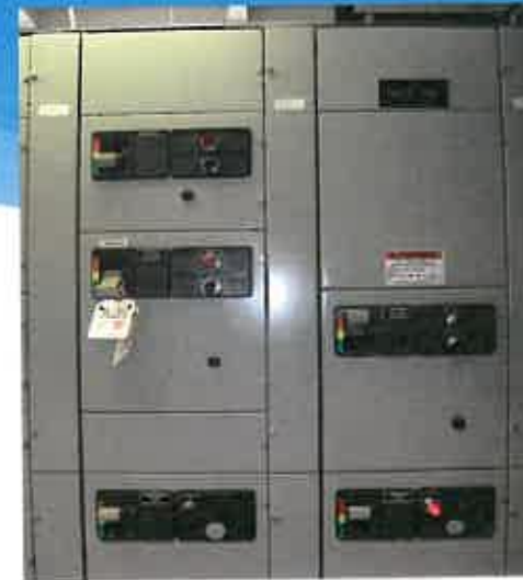
Switchgear at RP-1
