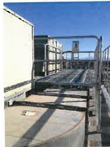
HVAC Unit Platform
