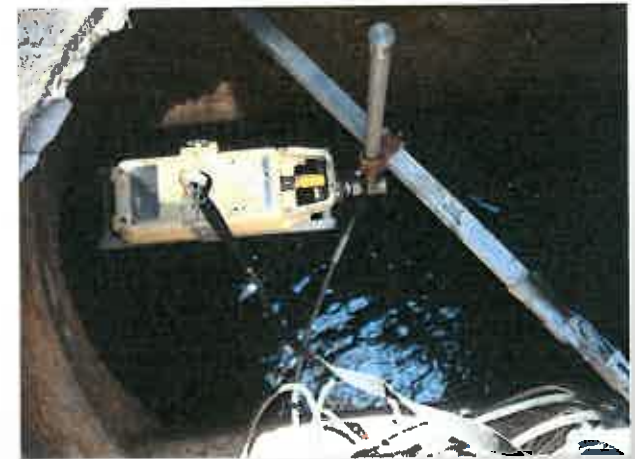
Existing Below Grade Sample Point
