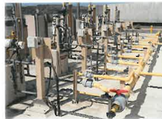
Sodium Hypochlorite Chemical Pumps
