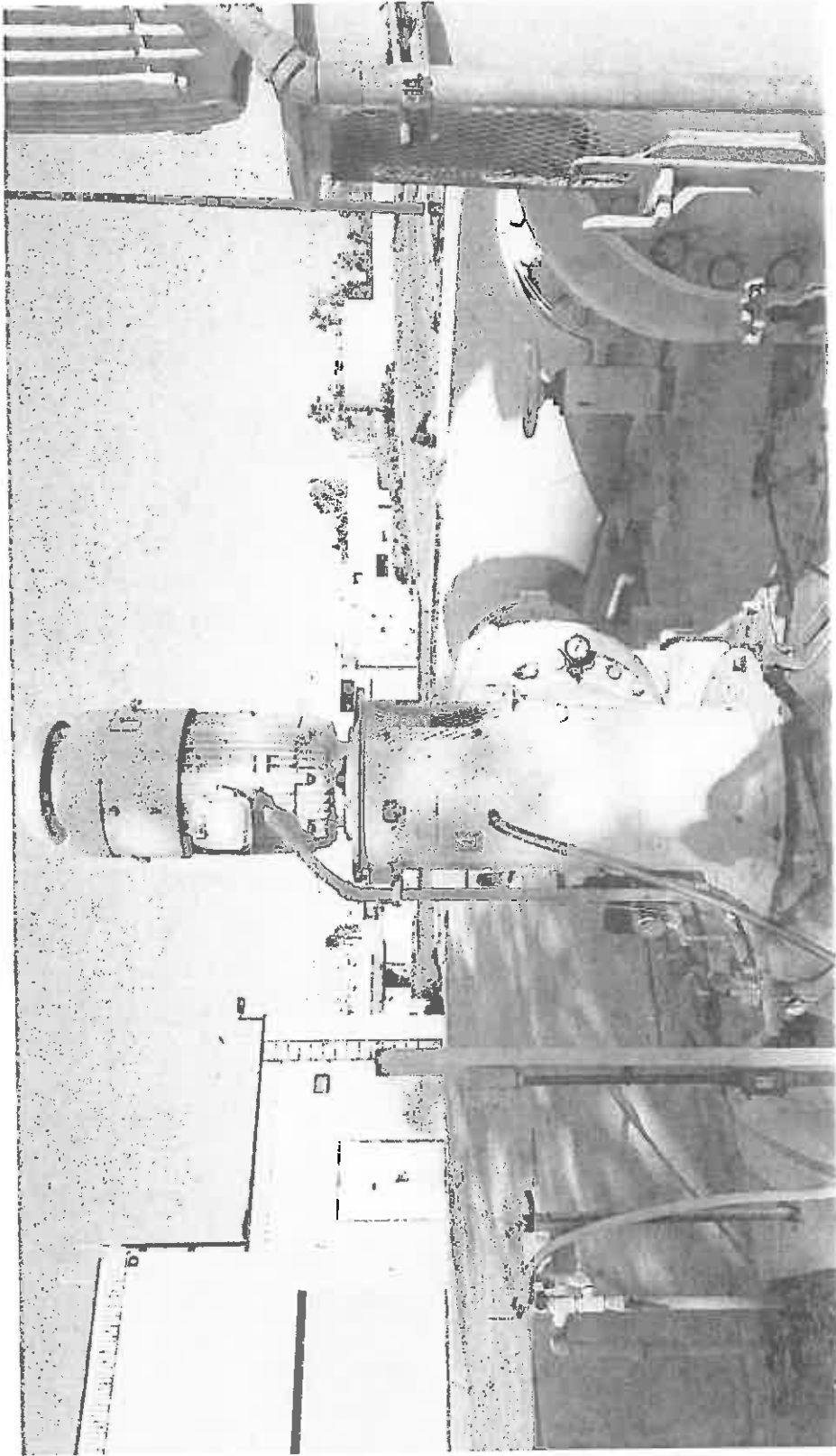
RP-1 Intermediate Pump Station Pump No. 1
