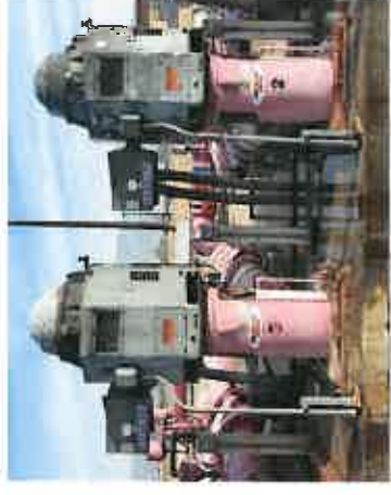
RP-1 1050 Pressure Zone Pumps 3 and 2 (61% and 63% Efficient respectively)
