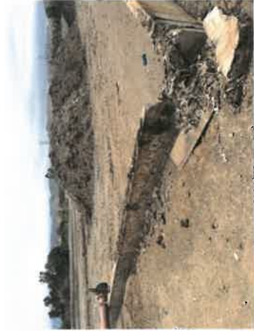
Failed Drying Bed Containment Wall to be Repaired
