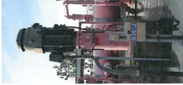
RP-1 930 Pressure Zone Pump No. 2 (51% Efficient)
