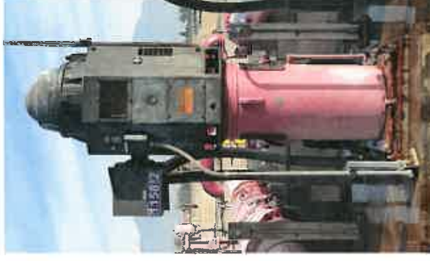
RP-1 1158 Pressure Zone Pump No. 2 (62% Efficient)
