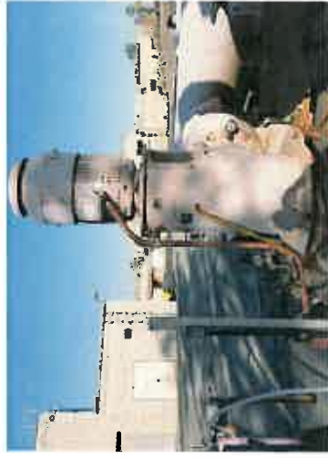
RP-1 Intermediate Pump Station Pump No. 1 (57% Efficient)
