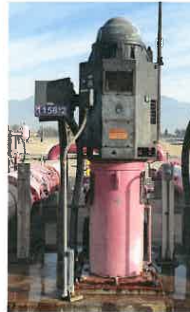
RP-1 1158 Pressure Zone Pump No. 2 (62% Efficient)
