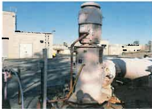
RP-1 Intermediate Pump Station Pump No. 1 (57% Efficient)
