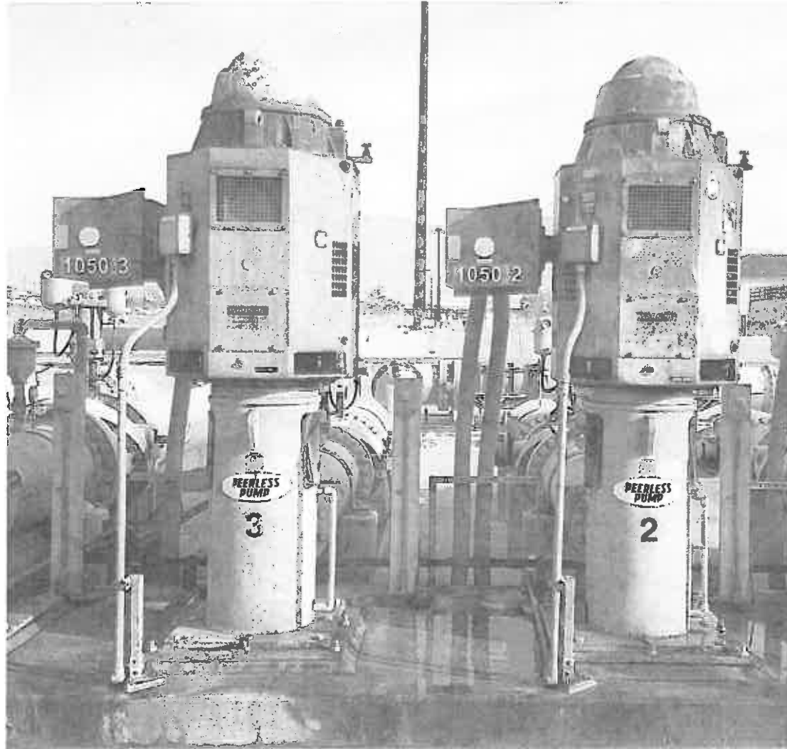
RP-1 1050 Pressure Zone Pumps No. 2 & 3
