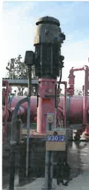
RP-1 930 Pressure Zone Pump No. 2 (51% Efficient)
