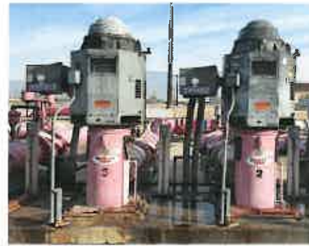
RP-1 1050 Pressure Zone Pumps 3 and 2 (61% and 63% Efficient respectively)
