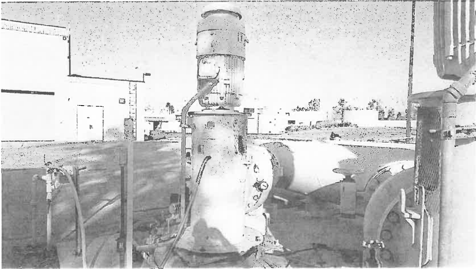
RP-1 Intermediate Pump Station Pump No. 1
