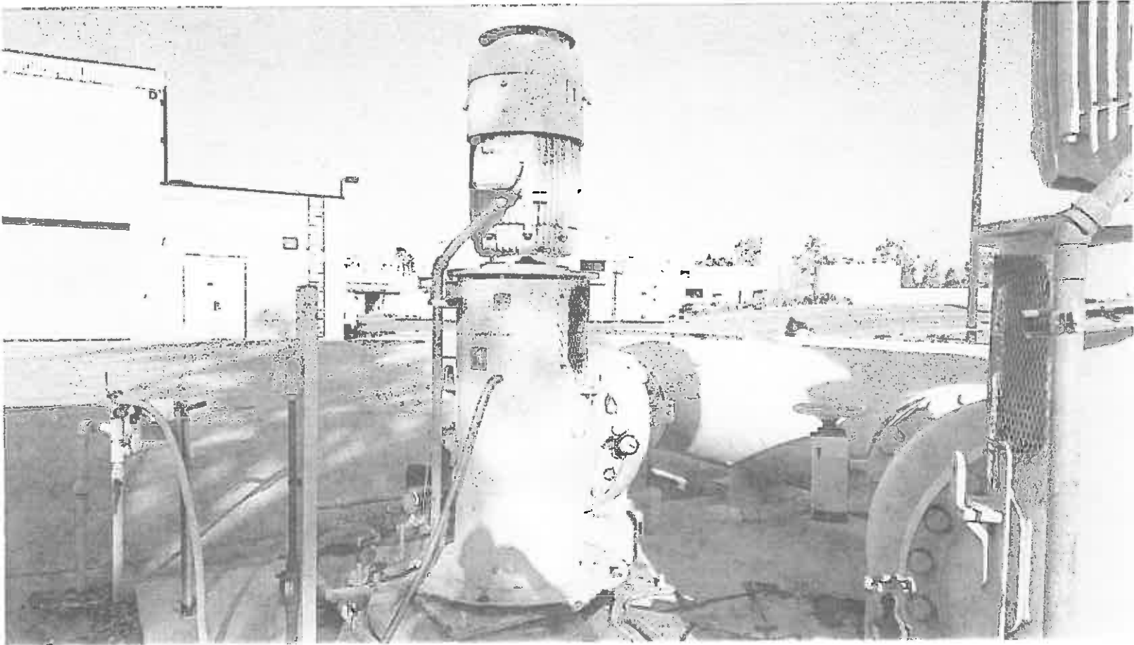
RP-1 Intermediate Pump Station Pump No. 1
