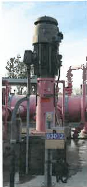
RP-1 930 Pressure Zone Pump No. 2 (51% Efficient)
