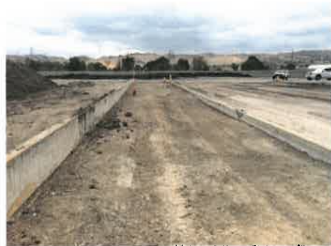
Access Road East of Plant to be Paved to New Storm Catchment
