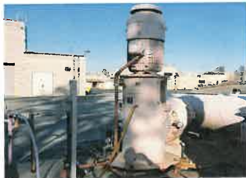
RP-1 Intermediate Pump Station Pump No. 1 (57% Efficient)
