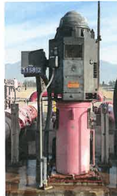
RP-1 1158 Pressure Zone Pump No. 2 (62% Efficient)
