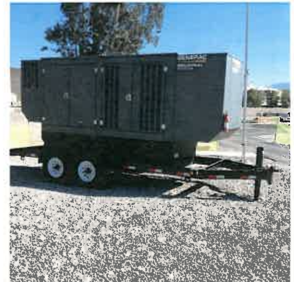
Existing Portable Generator
