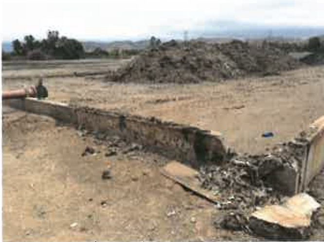
Failed Drying Bed Containment Wall to be Repaired
