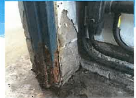
Corrosion Outside Containment Area
