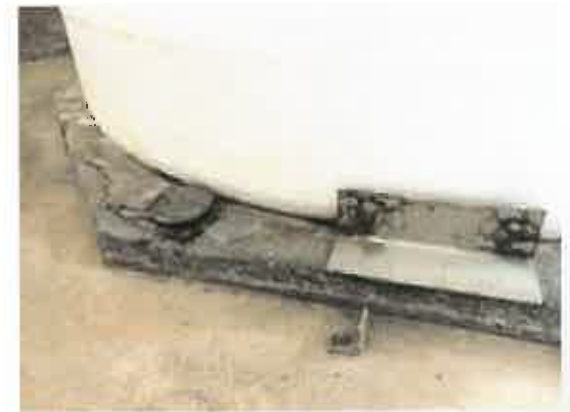
Damaged Concrete Pad Under Tank
