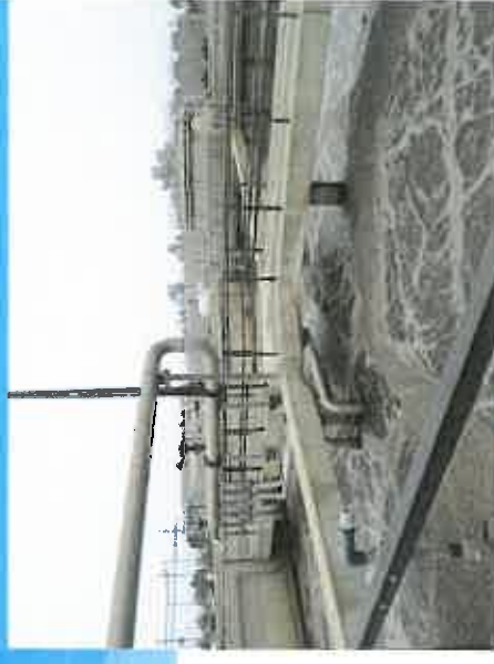
RP-1 Aeration Basins
