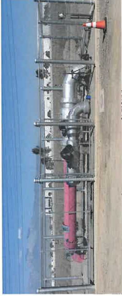
Valve Station at RP-3
