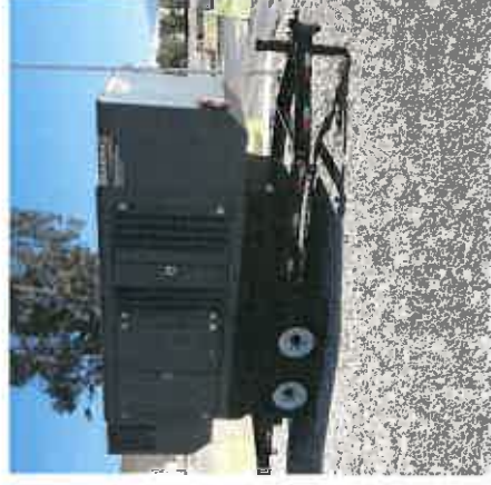
Existing Portable Genset
