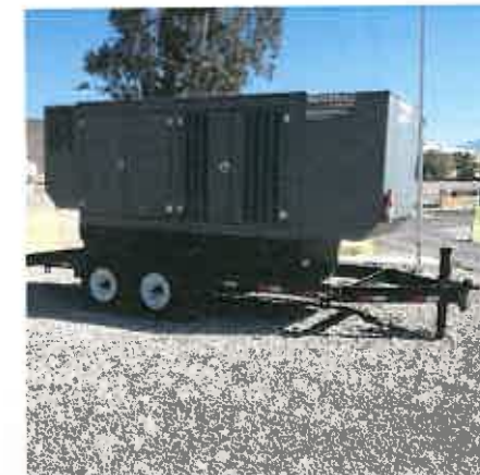
Existing Portable Genset
