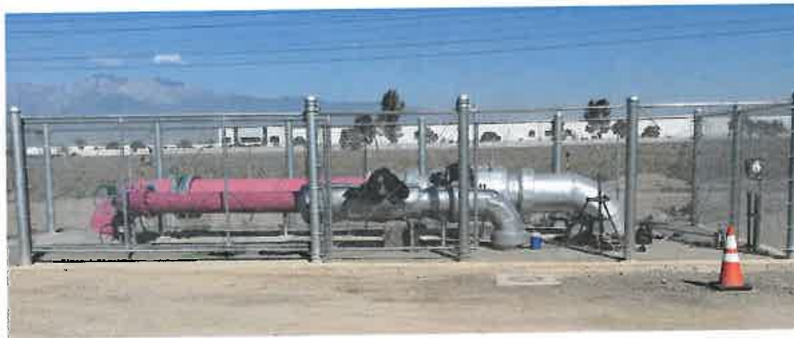
Valve Station at RP-3
