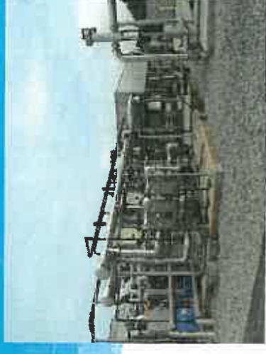
Central Chiller Plant
