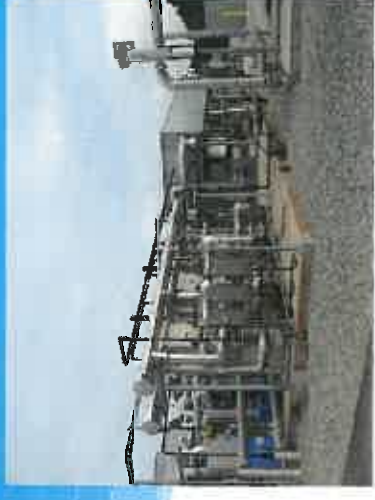
Central Chiller Plant
