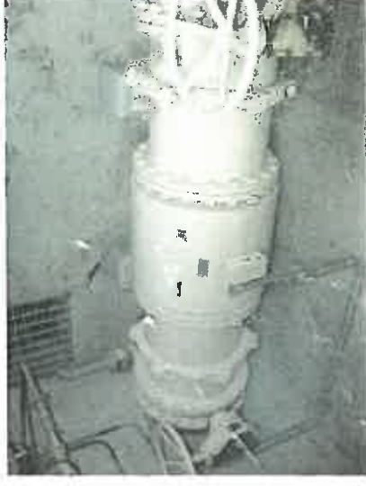
System C Flow Meter
