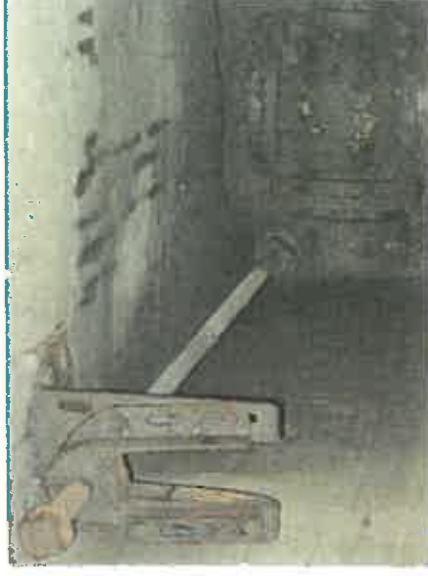
DAFT Valve Vault No. 2
