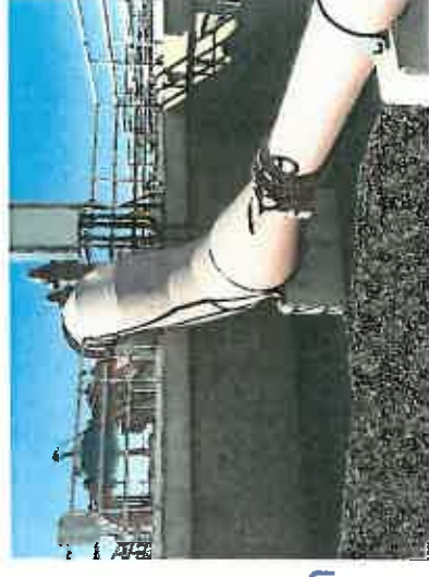
RP-5 RW Pump Station
