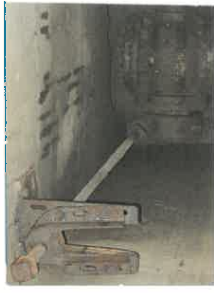
DAFT Valve Vault No. 2
