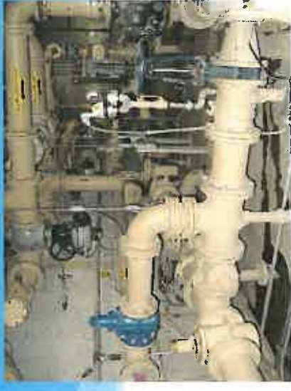
Scum Pump Location
