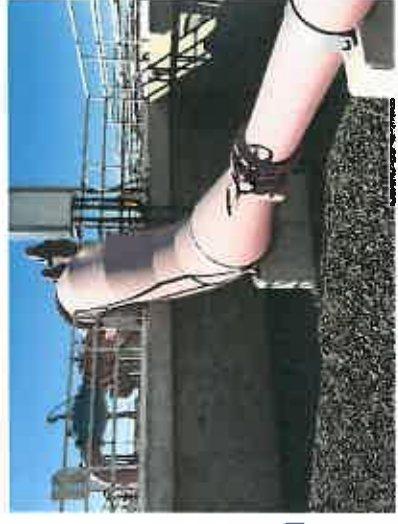
RP-5 RW Pump Station
