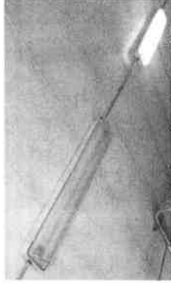
Existing 1x4x2 Vapor tight lights at RP-1 $65.00/year
