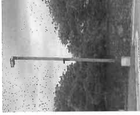
Existing 400W MH Arm Mounted Pole Street Lights at CCWRF $235.00/day
