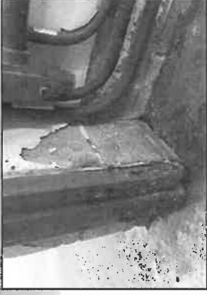
Corroded Existing at Chemical Building
