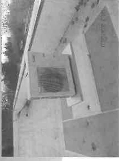
Condenser Unit at RP-5 Control Room
