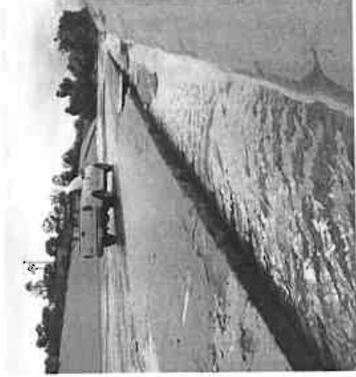
Slab Uplift Downstream of Trench
