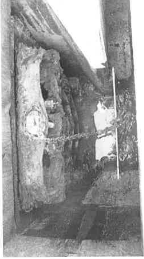
Cast Iron Sluice Gates are Obsolete and in-Operable
