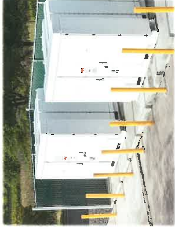
0.5 MW Tesla Battery Storage Installation
