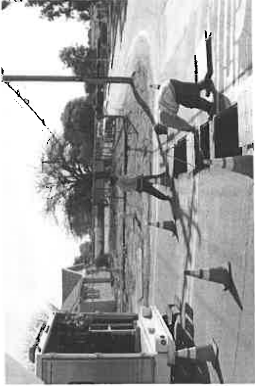
Removal of Access Covers is Time Consuming
