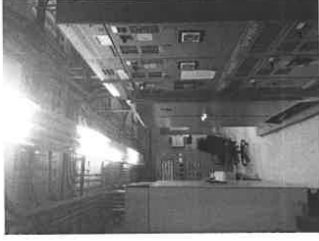
RP-5 Power Center No. 3
