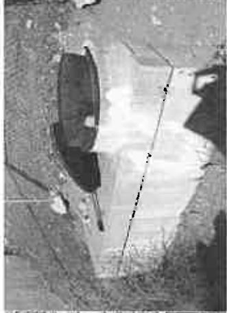
Inaccessible Manhole and Manhole Structure in the City of Chino Hills
