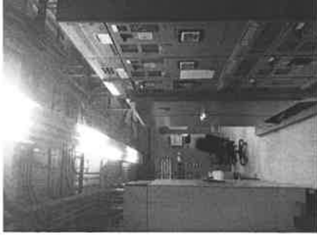
RP-5 Power Center No. 3
