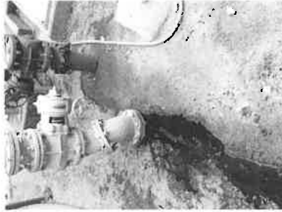
6-inch Sludge Line Leak
