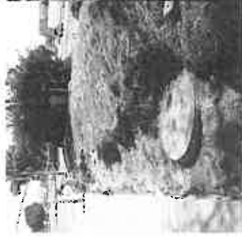
Deteriorated Manhole in the City of Ontario
