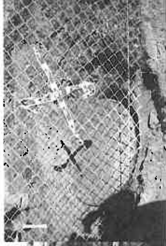
Deteriorated Manhole on Chino Basin Water Conservation District property
