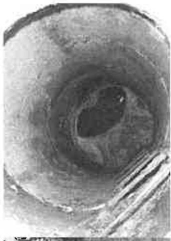
Deteriorated Manhole Shell in the City of Ontario
