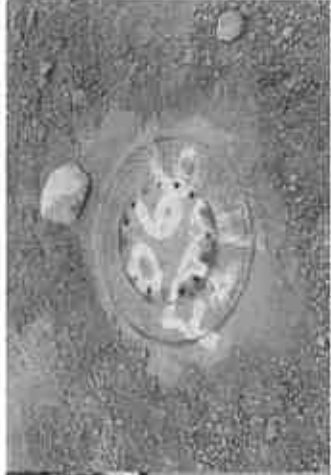
Buried Manhole on San Bernardino Flood Control property
