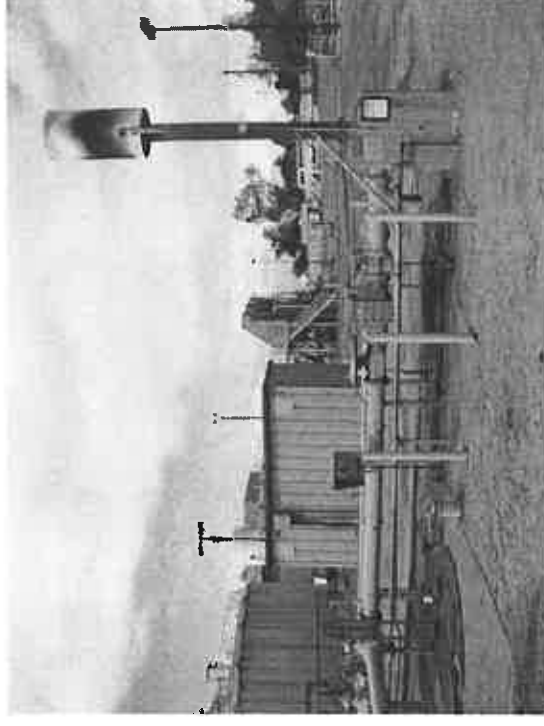
Existing Flare System
