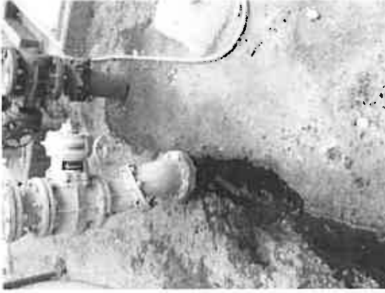
6-inch Sludge Line Leak
