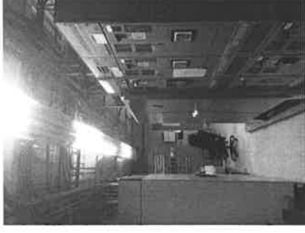
RP-5 Power Center No. 3
