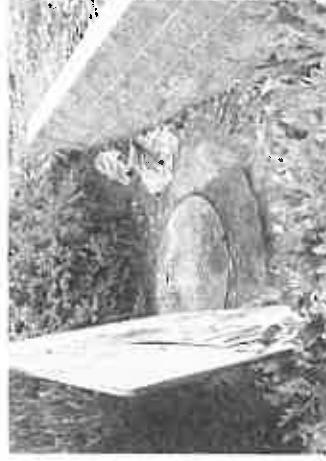
Inaccessible Manhole in the City of Chino
