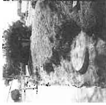
Deteriorated Manhole in the City of Ontario
