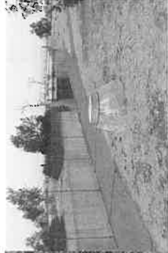
Inaccessible Manhole on San Bernardino Flood Control property
