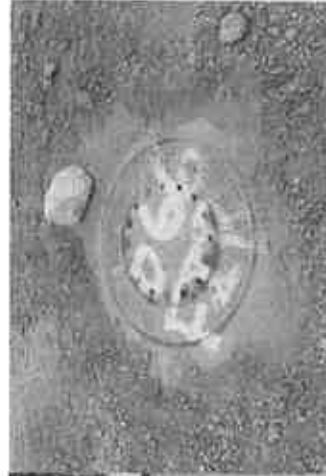
Buried Manhole on San Bernardino Flood Control property
