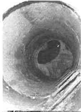
Deteriorated Manhole Shell in the City of Ontario
