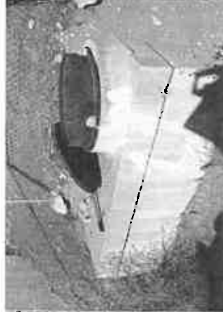
Inaccessible Manhole and Manhole Structure in the City of Chino Hills
