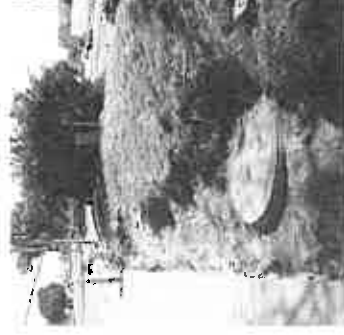
Deteriorated Manhole in the City of Ontario
