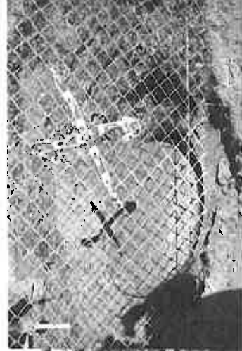
Deteriorated Manhole on Chino Basin Water Conservation District property
