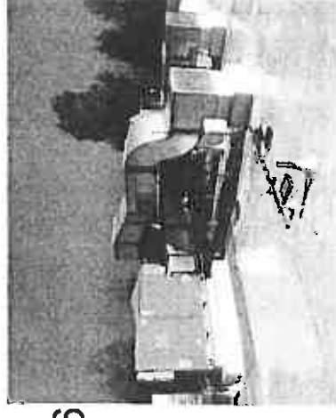
RP-5 Control & Server Rooms HVAC
