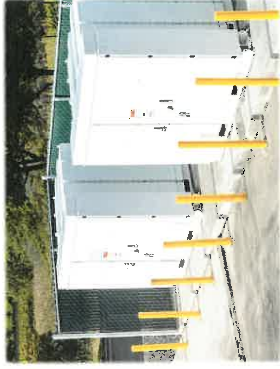
0.5 MW Tesla Battery Storage Installation
