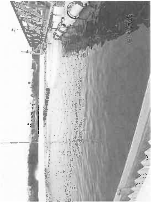
Clarifier No.3 ready for operation
