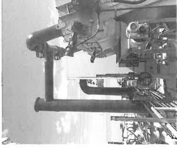
Backside of New Screening Process
